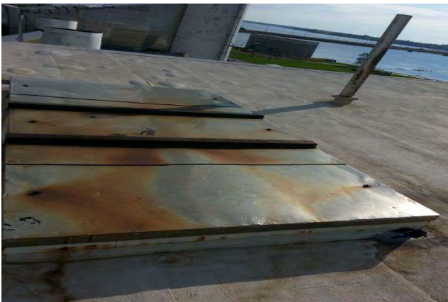
Low flashing height at cap unit.
