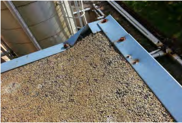
Poor metal counter flashing detail at perimeter.
