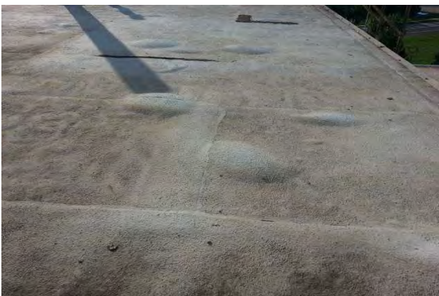
Blisters visible on roof membrane.
