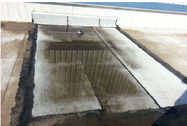
Visible ponding water overtop previous roof repair.
