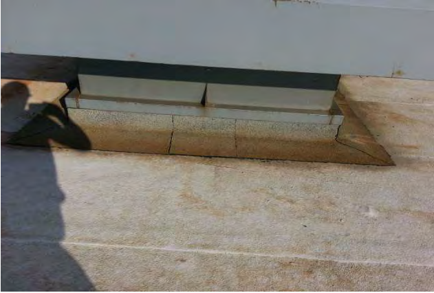
Low flashing height at curb unit. Proper flashing detail is minimum 8in above roof surface.
