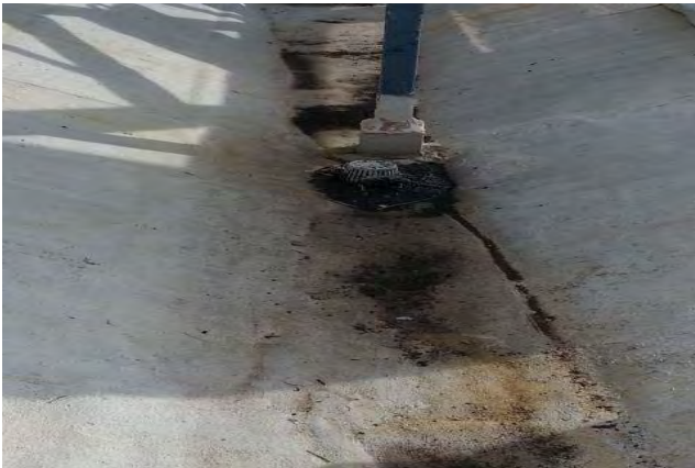
Debris visible around drain area.
