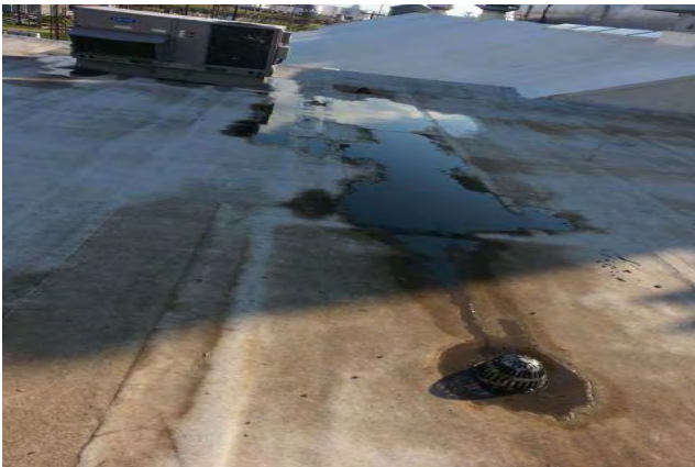
Visible ponding water overtop roof system. Water pouring out of hvac unit is not slopping to drain.
