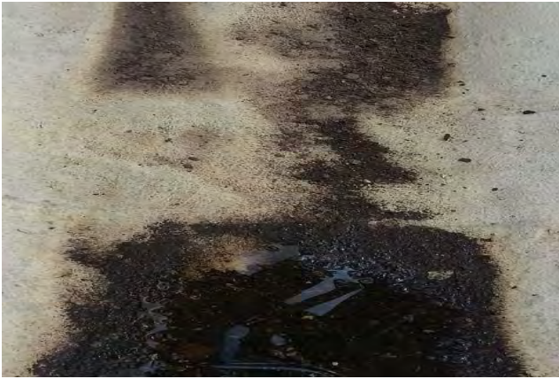
Debris visible at valley
