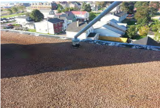
South corner pitch pan requires attention. Fall arrest work plan will be required.
