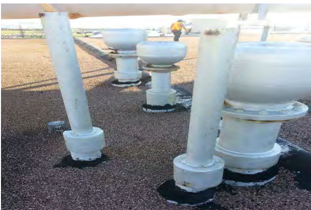
View of soil stack and vent units. All mastic at flashing requires attention.
