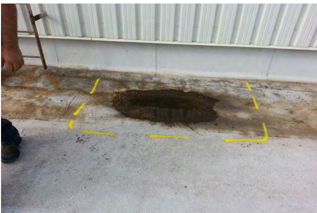
Test cut indicates @ 9 sq ft of wet insulation
