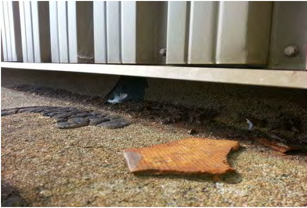
Open lap seam at perimeter.
