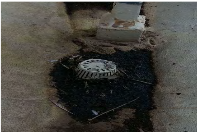
Debris visible around drain area.
