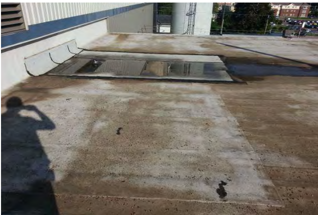
Visible ponding water overtop previous roof repair.
