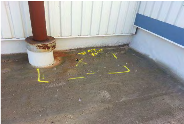
Thermal scan identified @ 10 sq ft of wet felts within roof area.
