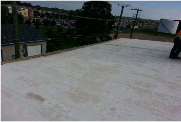
Poor quality drip edge detail affecting exterior drainage system. Deteriorating restorative coating at roof perimeter.
