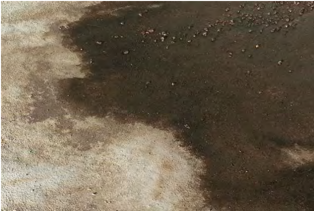
Noticeable staining and granular loss on modified bitumen membrane.
