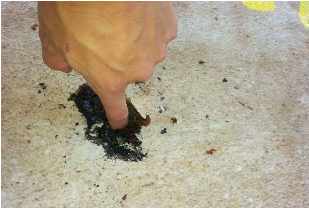
Verification cut indicates wet insulation.
