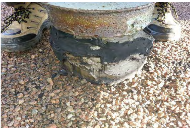
Chimney unit pitch pan requires attention.
