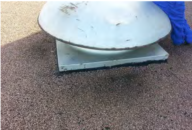
Low vent unit flashing height. Flashing curb should be minimum 8in above roof surface.
