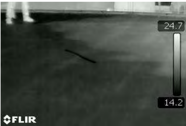
Thermogram photo # 3 identified @ 226 sq ft of wet insulation.
