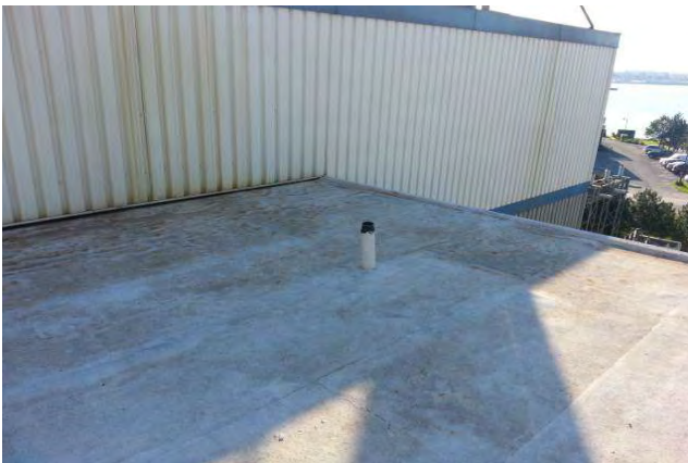
Visible granular loss on roof membrane.
