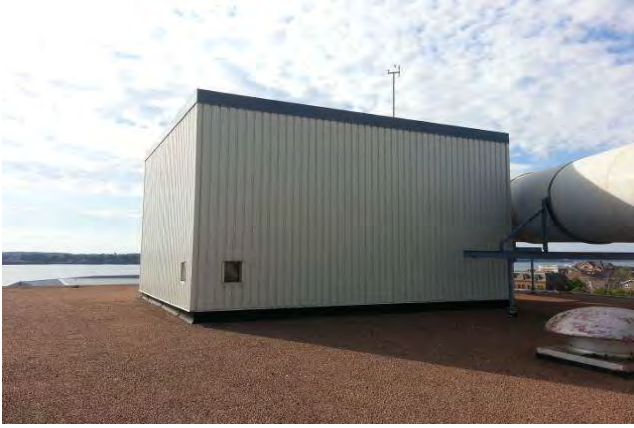
Roof view. No ladder access to roof unit.
