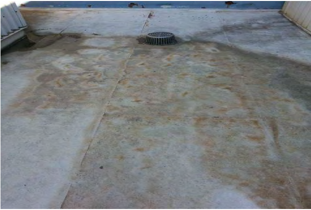
Noticeable staining and granular loss on modified bitumen membrane near roof drain.
