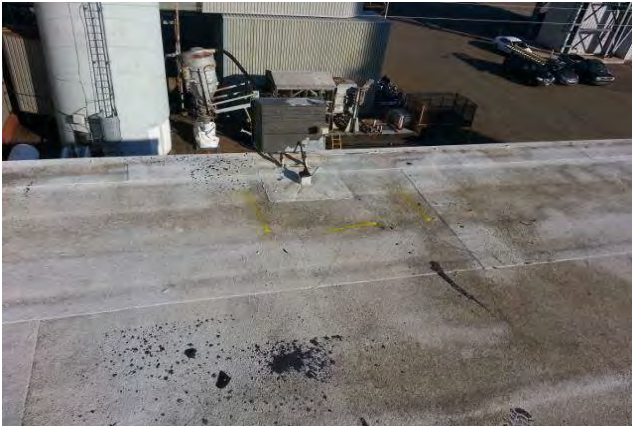
Thermal scan identified @9 sq ft of wet within system. Fall arrest work plan will be necessary.
