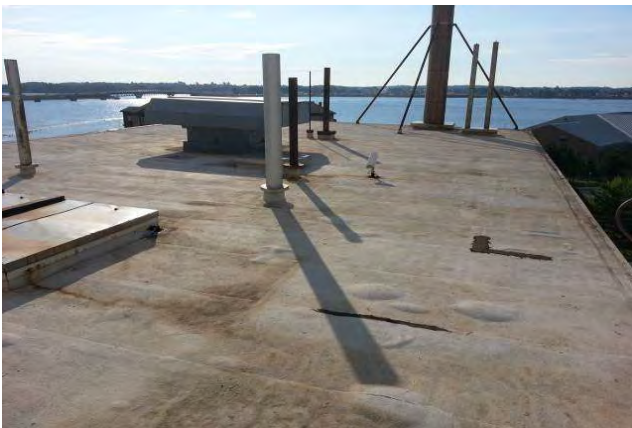
Roof view. Blisters visible on roof membrane.
