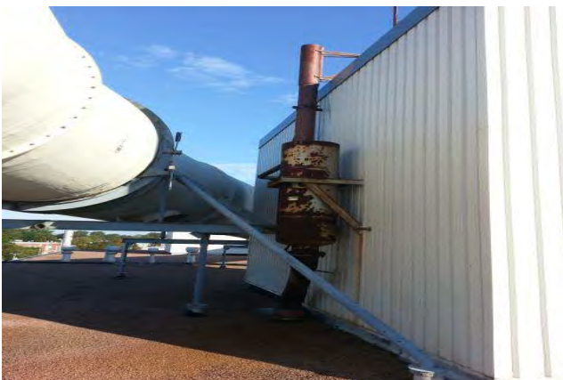
North west corner chimney unit is corroding.
