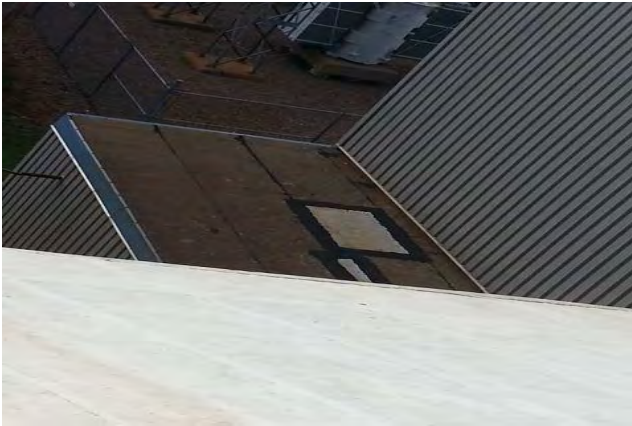
Roof view. Previous repairs are visible.
