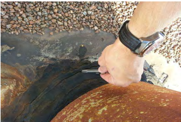
Chimney unit mastic requires attention.
