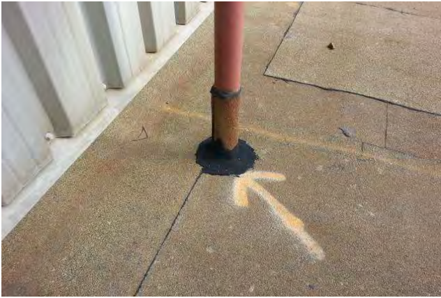
Mastic at soil stack needs to be addressed.
