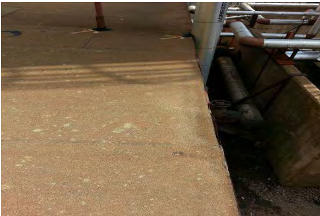
Roof gravel stop detail is completely deteriorated. Water can infiltrate roof system.
