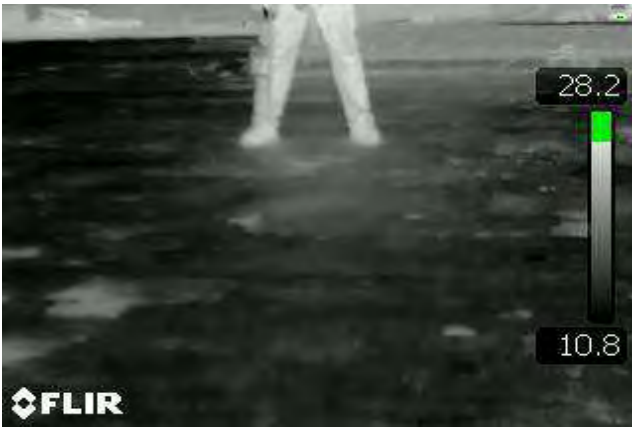
Thermogram photo #1 indicating dry insulation throughout roof membrane.
