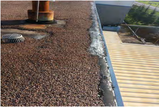
South perimeter gravel stop caulking requires attention.
