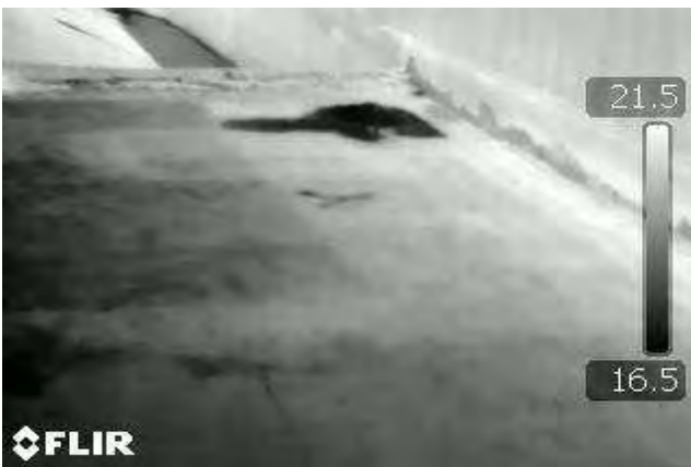
Thermal scan photo #4 identified @ 90 sq ft of wet insulation.
