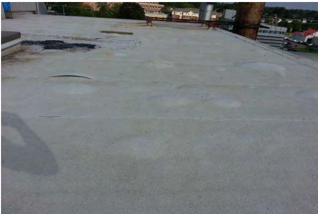
Blisters visible throughout roof membrane.
