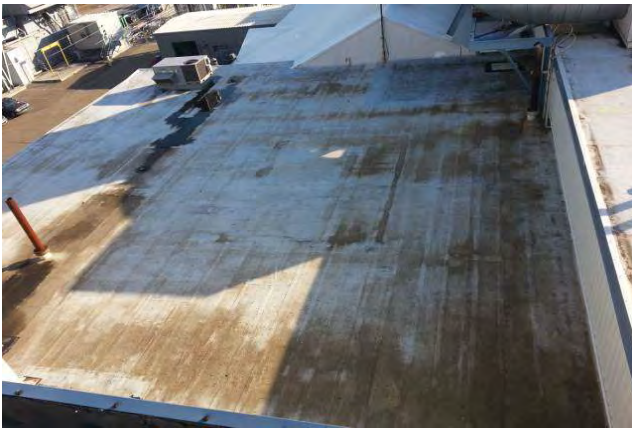
Roof view. Visible staining and granular loss on roof membrane.
