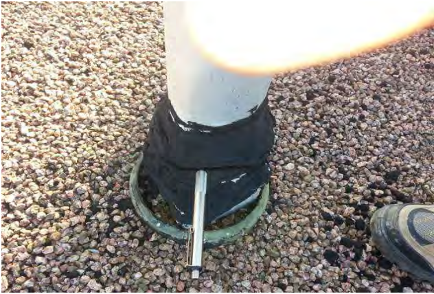
Soil stack mastic requires attention.
