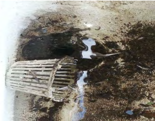
Clogged drain. All debris should be cleaned off roof area.
