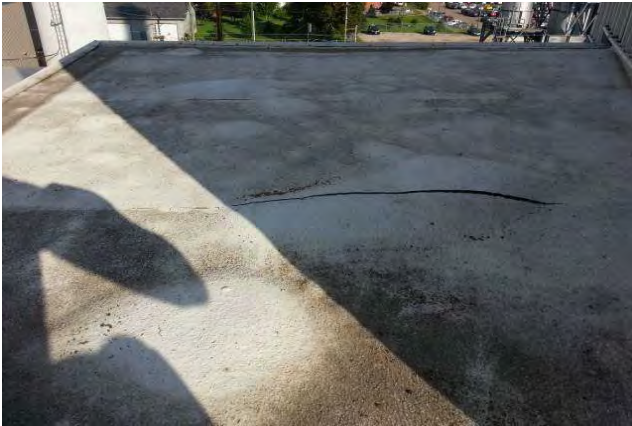
Large blisters visible on roof membrane.
