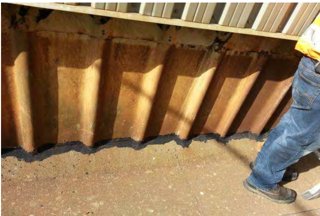
Poor flashing detail at South wall. Low flashing height and mastic is deteriorating.
