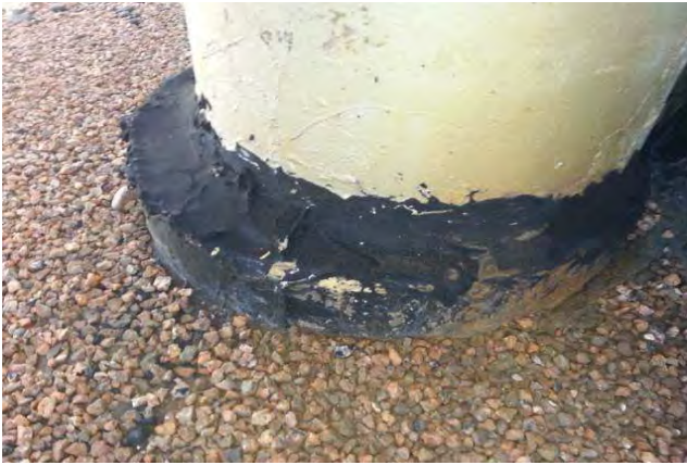
Chimney unit pitch pan requires attention.
