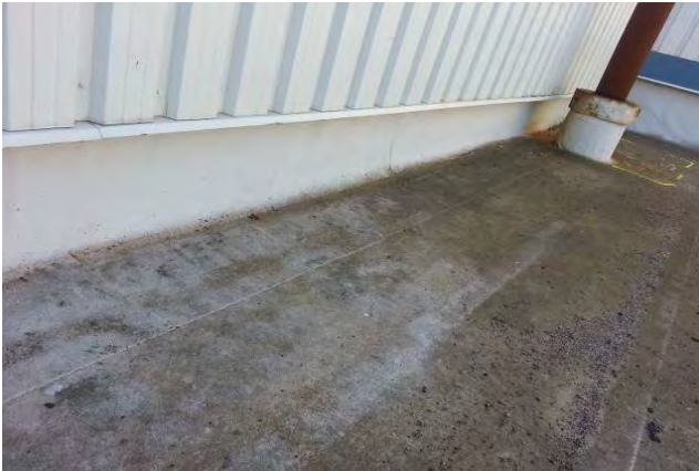
Visible staining and granular loss on roof membrane.
