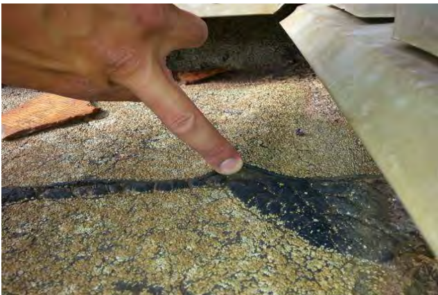
Open lap seam at perimeter.
