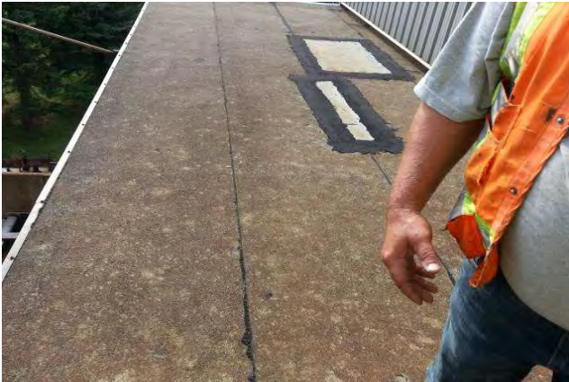
Roof view. Previous repairs are visible.
