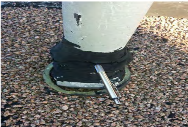
Soil stack mastic requires attention.
