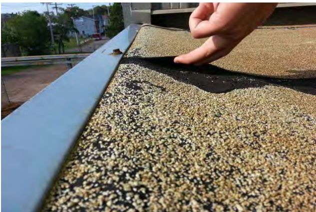
Open lap seam at perimeter.
