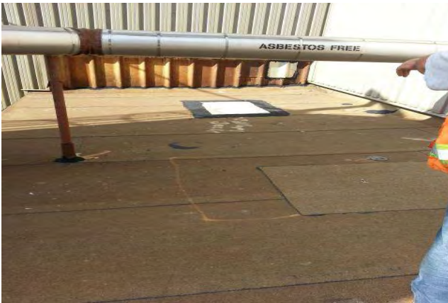
Roof view. Previous repairs visible.
