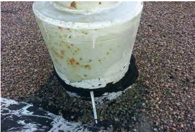
Soil stack mastic requires attention.
