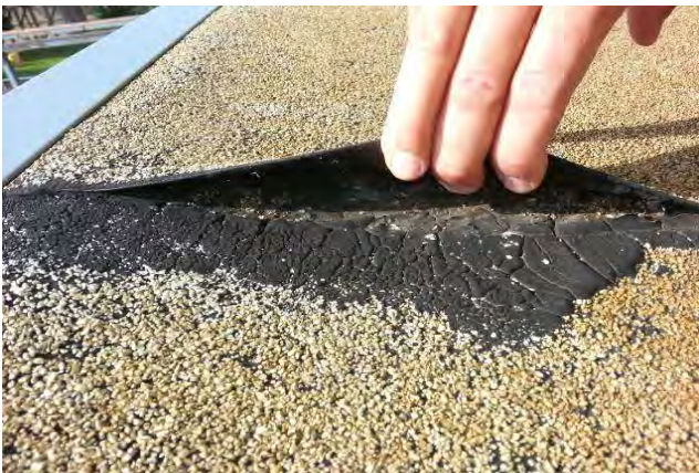
Open lap seam at perimeter.
