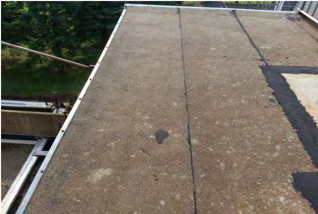
Granular loss on roof membrane is visible.
