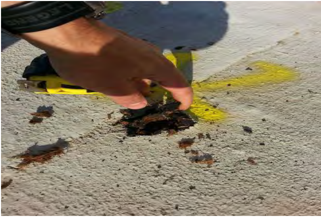
Test cut identifies wet insulation.
