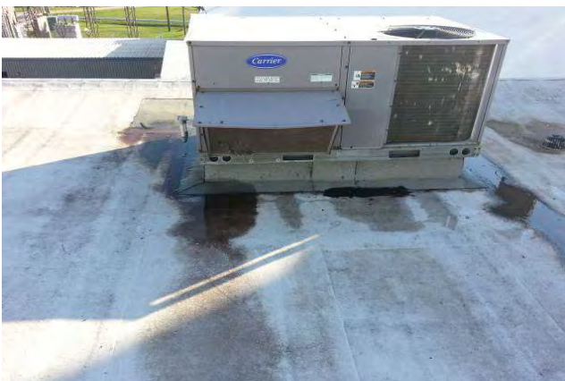
Water pouring out of hvac unit is not slopping to drain.
