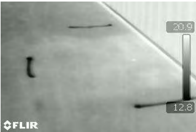
Thermogram photo # 2 identified @ 28 sq ft of wet insulation.
