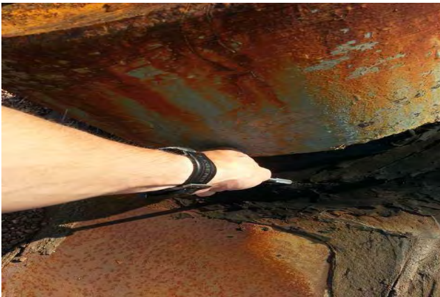
Chimney unit mastic requires attention.
