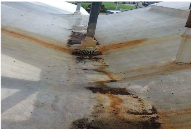
Debris visible at valley
