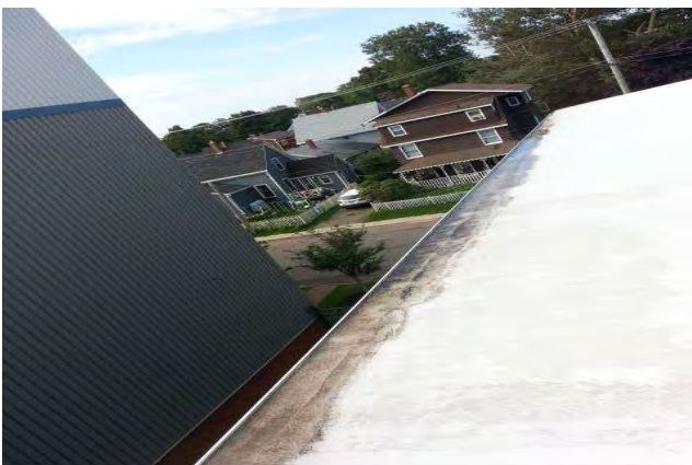
Poor quality drip edge detail affecting exterior drainage system. Deteriorating restorative coating at roof perimeter.
