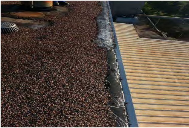
Roof view. Some corrosion visible on metal roof membrane.
