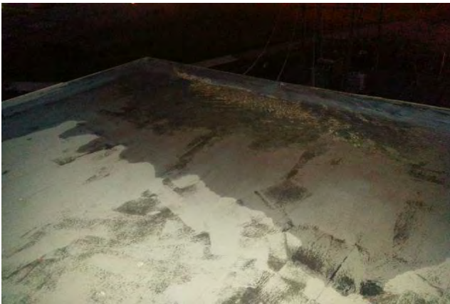
Minor water visible at SW perimeter. As rainfall was within 24h, ponding water cannot be confirmed.
