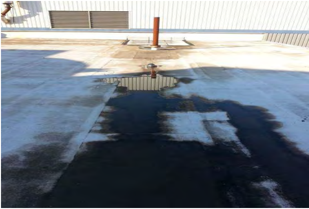
Noticeable staining and granular loss on modified bitumen membrane near roof drain.
