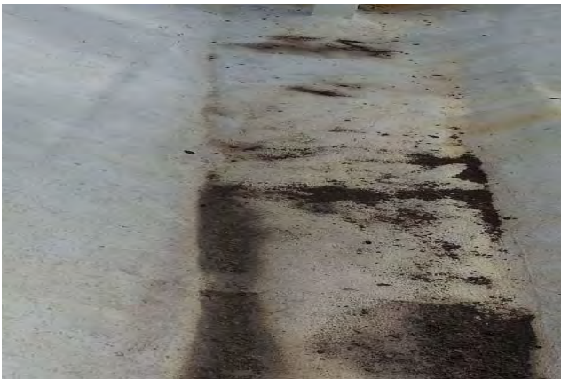
Debris visible at valley
