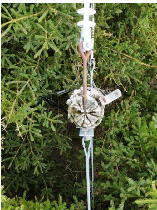
Deteriorated pole top with primary hardware exposed.
