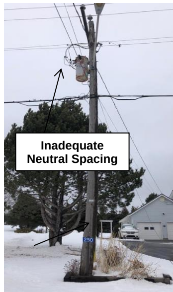
Figure 3 Inadequate neutral spacing and rusted transformer.
