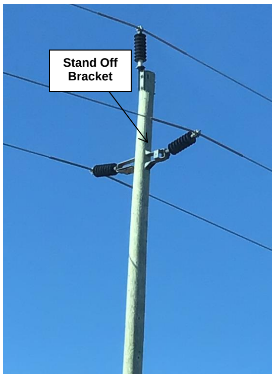
Stand-off brackets on insulator to be replaced.
