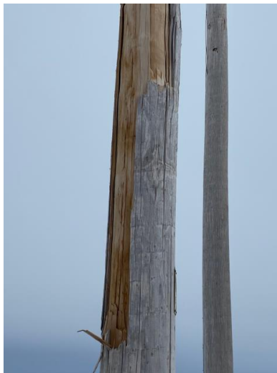
Wood is splitting on pole.
