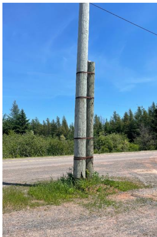
Cracked, damaged pole.
