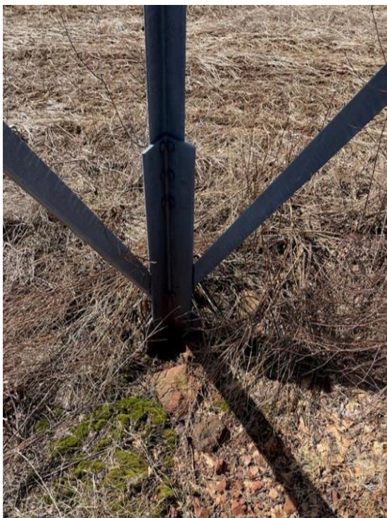
Sunken tower base.
