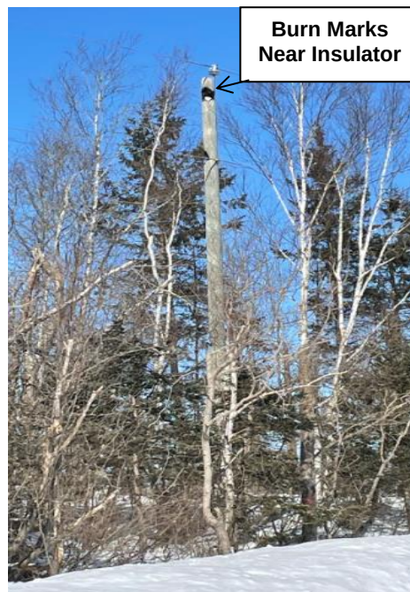
Burn marks from a failed insulator.
