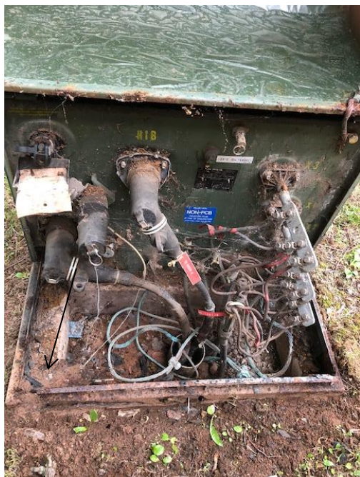
Rusted padmount transformer with sunken concrete pad.
