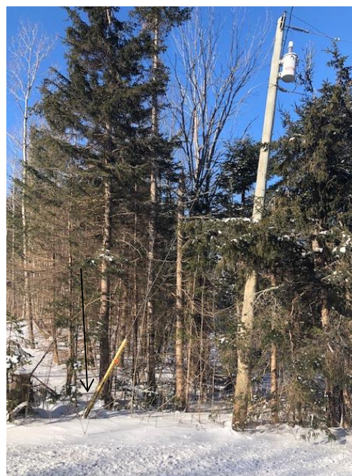
Slack anchor allowing the pole to lean.
