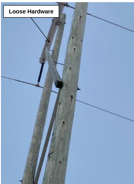
X-brace detaching from pole.
