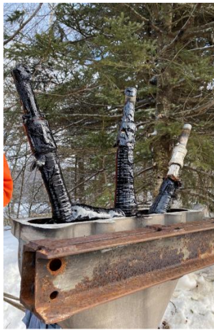
FIGURE 5 Cable Termination Failure
