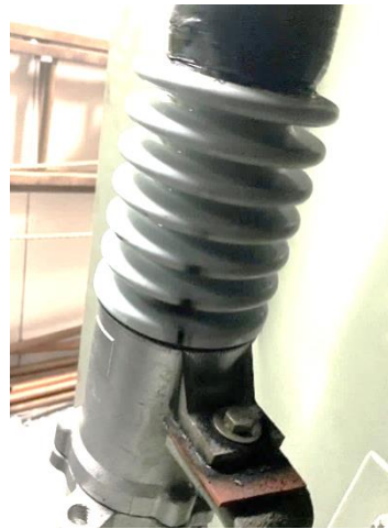
FIGURE 6 Arcing Failure within the 13.8kV Switchgear
