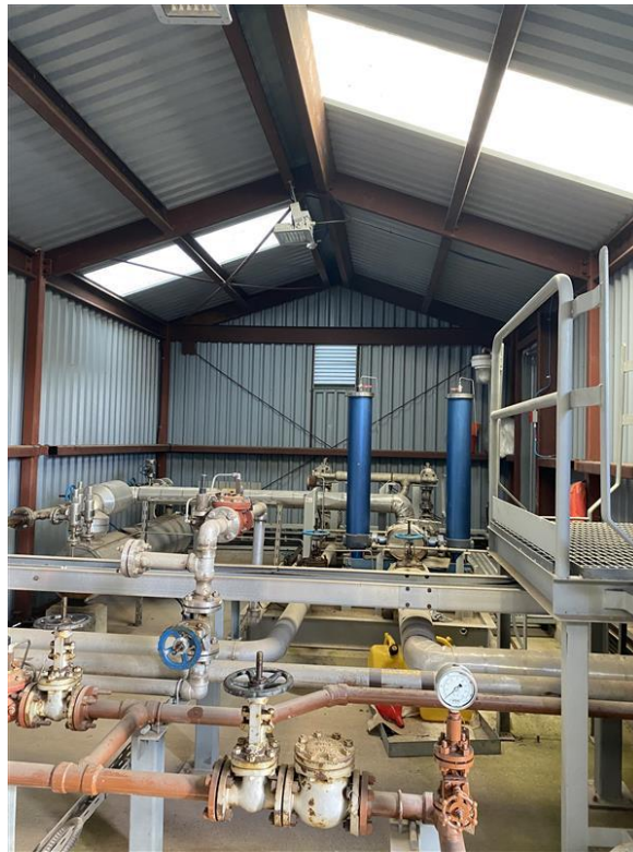
FIGURE IR-1(iv) Fuel Forwarding Equipment Enclosure Interior
